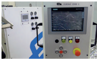
Main operating panel.
